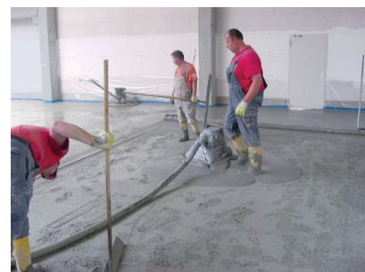
Application with pneumatic conveyor
