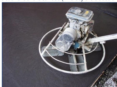
Picture 9: Smoothing of hard aggregate layer with power trowel (blade) (concrete finisher)
